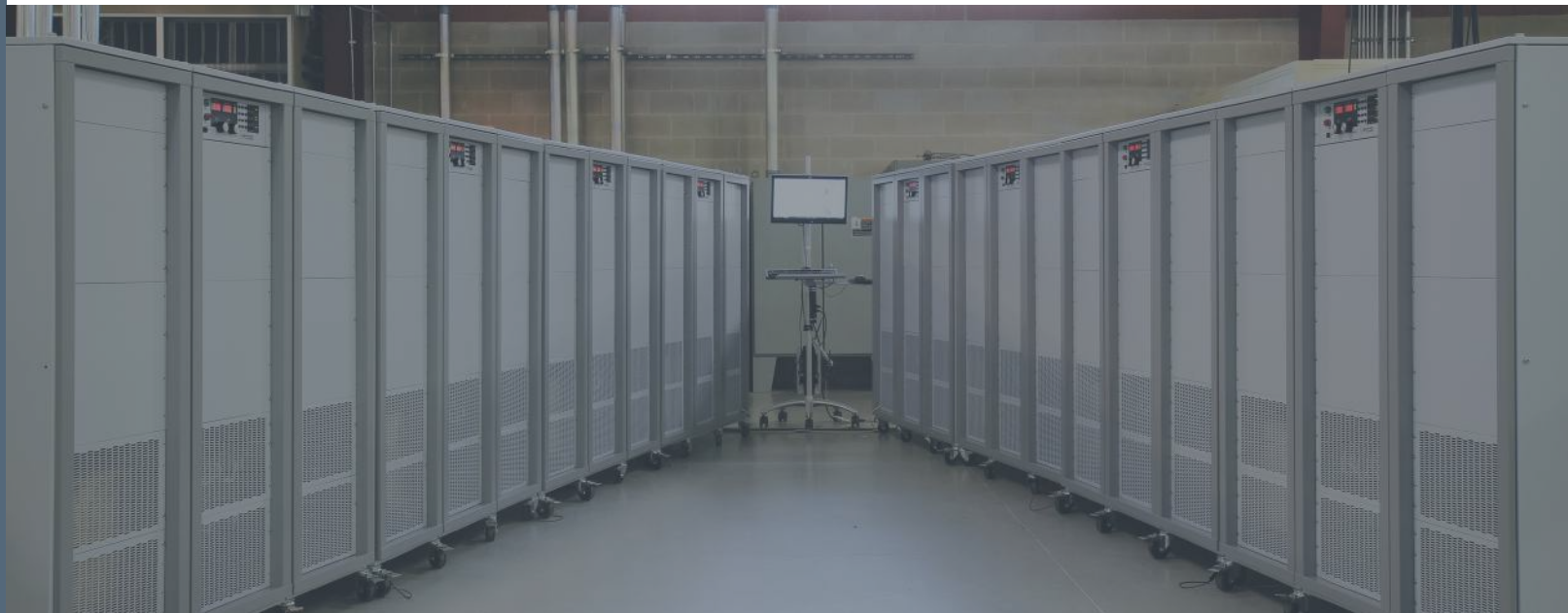
Qty (8) 250 kW MT Series units in master-slave parallel to form a 2 MW system
